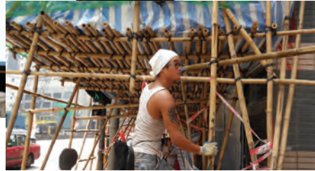
Image source: Wikimedia: Construction worker building a bamboo scaffolding in Hong Kong
